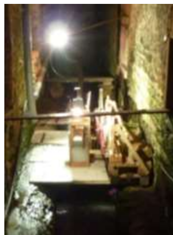
The functioning turbine
